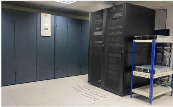
DATA CENTER HQ ML&C Rwp
